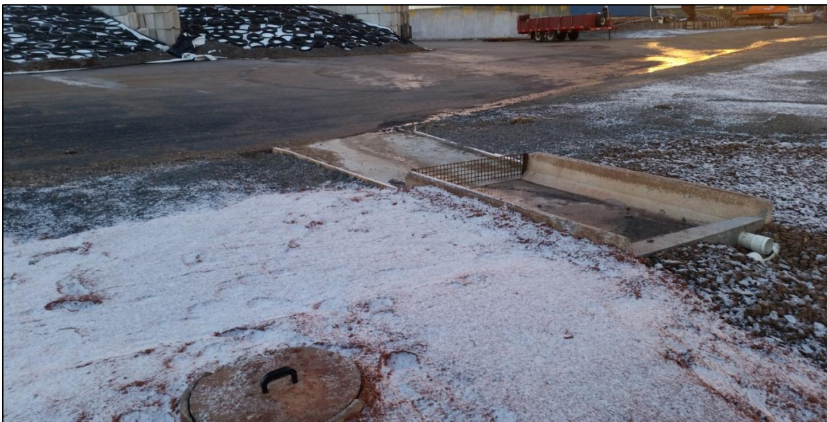
Figure 1: System is designed for any silage seepage to flow to the collection pit and into the storage tank
