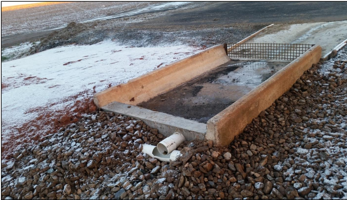
Figure 2: Screen filter, collection pit and diversion pipe
