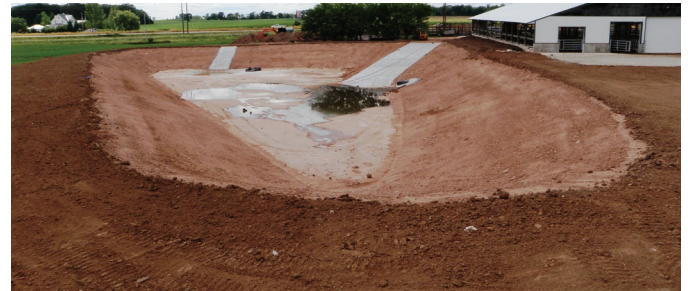
Figure 1: Earthen manure storage with clay liner showing concrete ramps and erosion protection. Image source: Winnebago County Land & Water Conservation Department (Used with permission)
